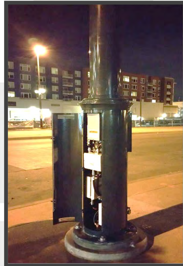
Equipment Inside of Pole Base
